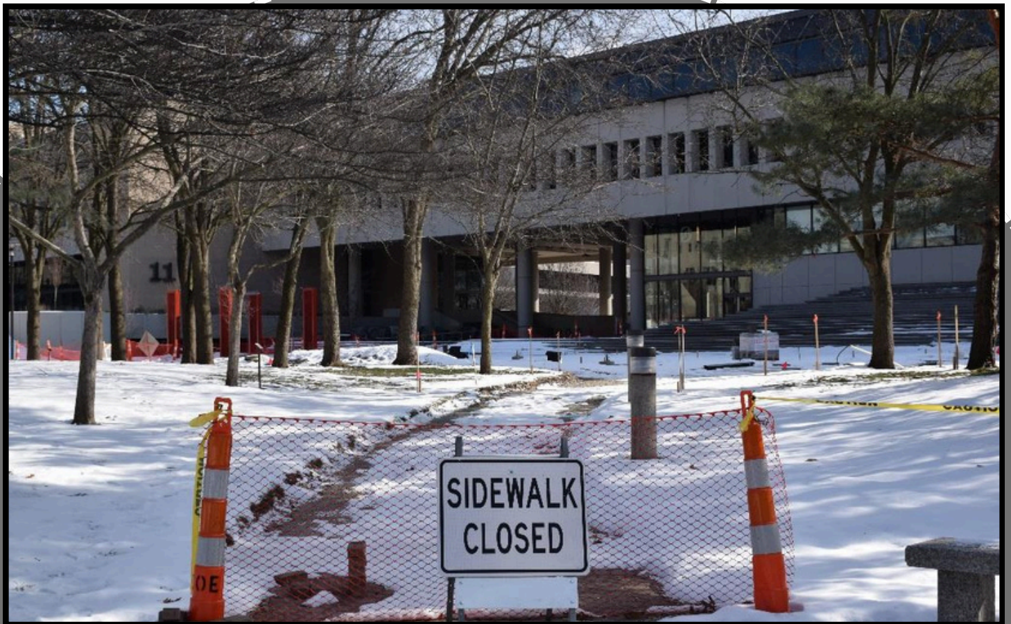
The construction of the sidewalk at Sinclair campus. Photo Provided by: Noah Schlarman
